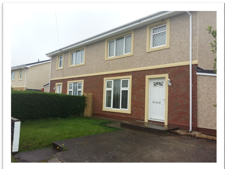
Completed properties at Gendros Avenue East, Swansea. Works included Roofing, Fascias, Rainwater Goods, EWI, Kitchens, Bathrooms, Electrical Rewiring, External Works, internal Alterations & Redecoration, Disabled Adaptation Works.
